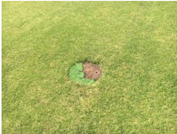
Picture 3 Cover on quick coupling valve
