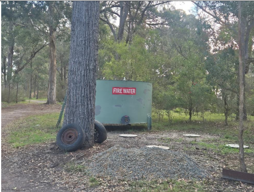
Existing water tank for fire fighting
