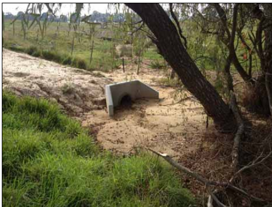
Figure 4-5 Example of high sediment load to a natural waterway
