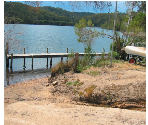
Erosion due to storm water flows
