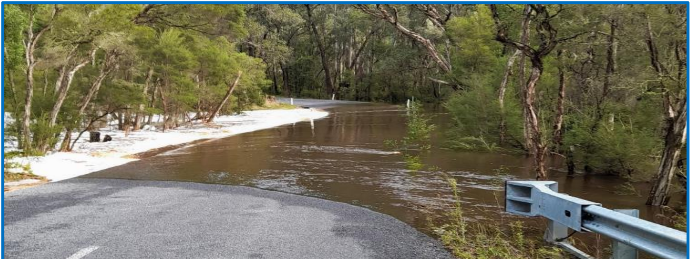
Scriveners Road Lakes Entrance is prone to flooding
