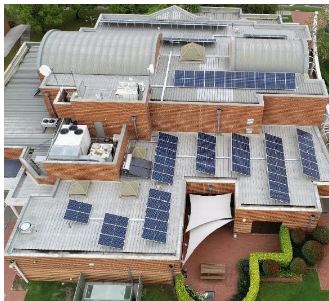
5. Main Corporate Centre & Council Chambers, 26 kW
