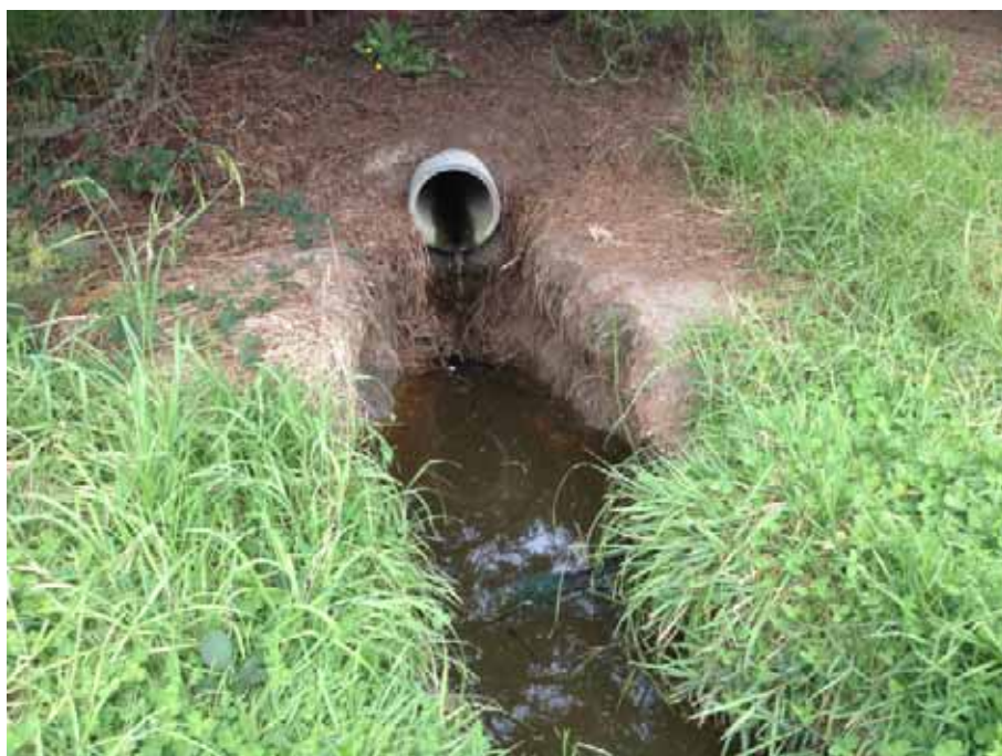
Figure 5-4 Direct discharge to the creek of stormwater without adequate headwall protection
