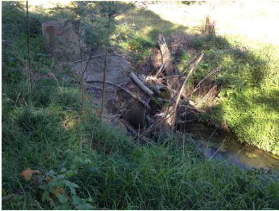
Figure 5-7 Stormwater pipe inlet/barrier
